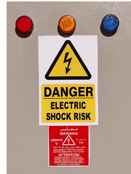
Figure G.28 Typical electrical warning label
