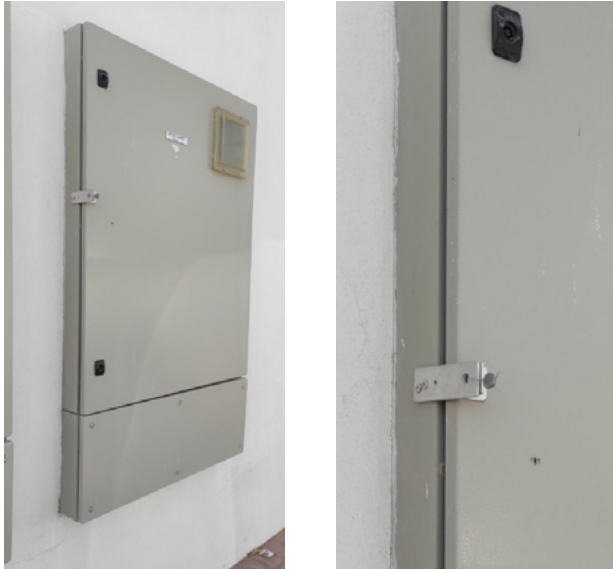
Figure G.9 Typical metering cabinet padlocking and wire tag
