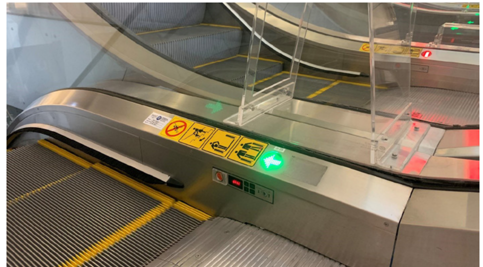
Figure D.2 Escalator with detectors at top and bottom landing areas
