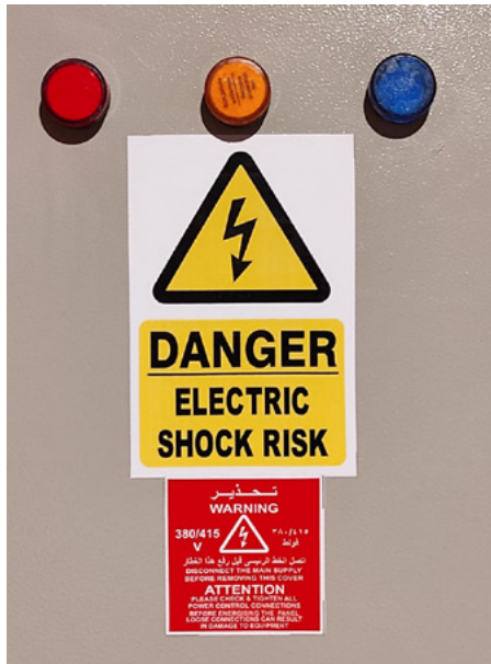
Figure K.81 Typical electrical warning label
